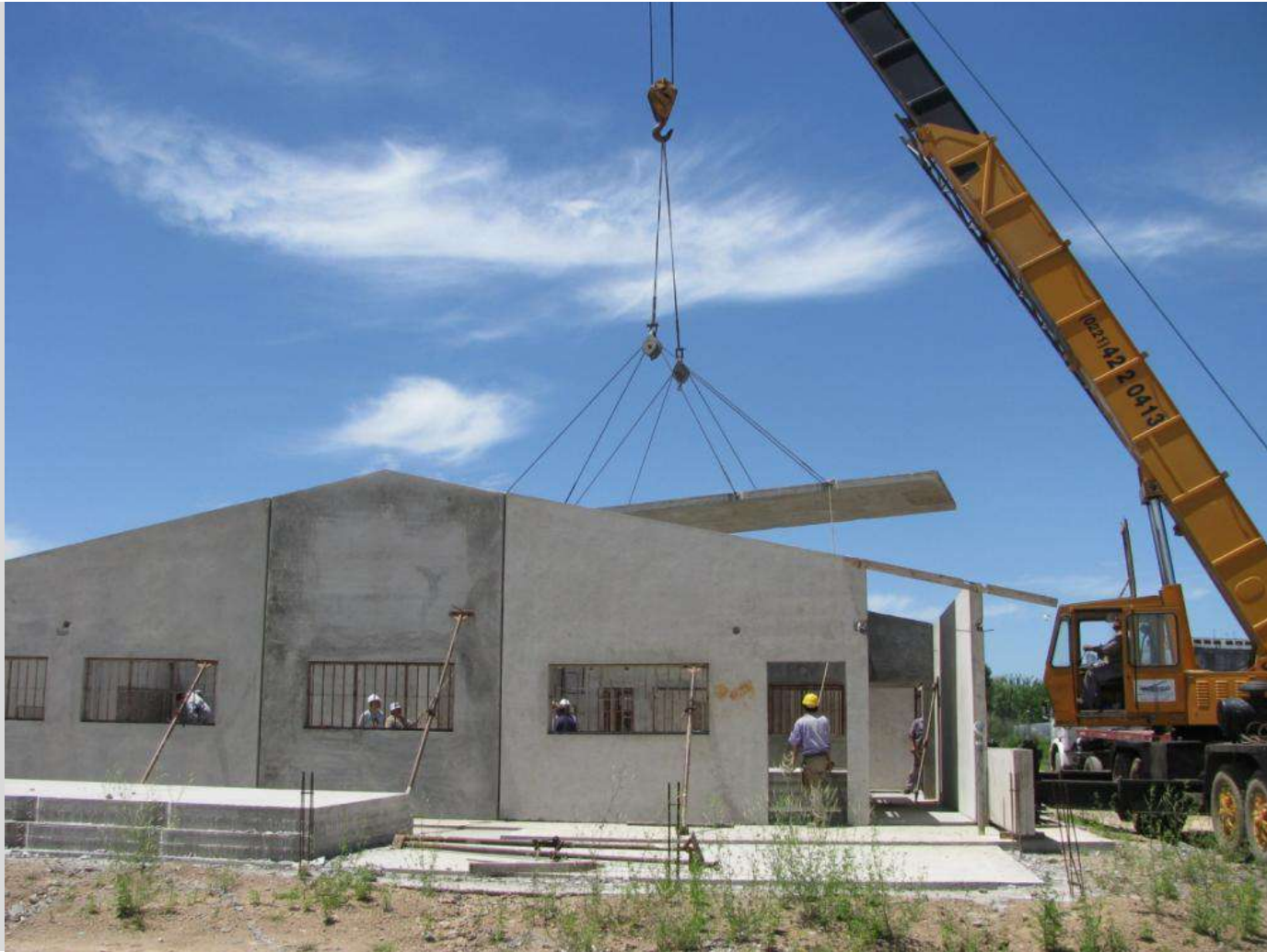
Olmos Prison, Provincia de Buenos Aires, Argentina Applied system: On site Precasts. Area: 10.000 m 2
